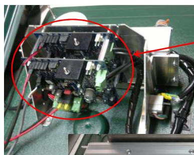
Multiple Station boards
